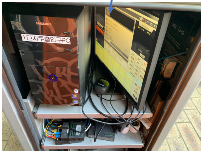
Third-party license plate number reader configuration: PC for vehicle number recognition (1) + vehicle number reader camera, lighting, control board (2) + vehicle circuit breaker (3)
